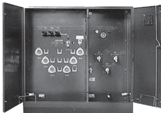
Fig. 1.26 Transformador de pedestal (Pad Mounted)
